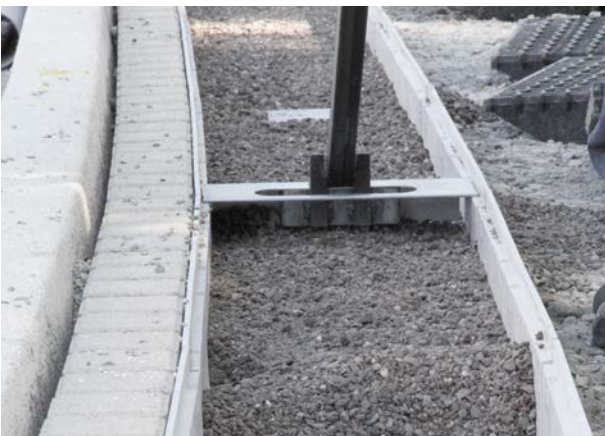
Step 3: Filling in and level-off the second substrate layer "Biocalith MR-F1" with the use of the MEA level-off gauge.
