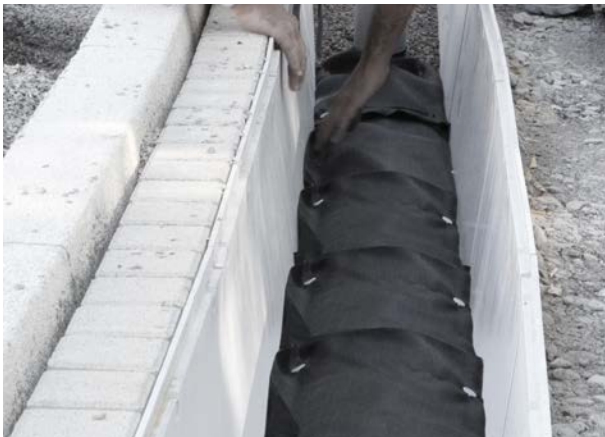
Step 1: Insertion of the spacers covered with geotextile in the laid down gutter strands
